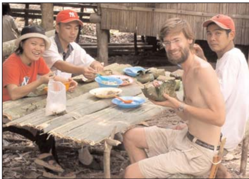
Dodger Stirling (center right) enjoys his lunch break with Terian residents during construction of the hydro catchment system. The bamboo table and benches they are using were made in the same time it took to prepare lunch!
